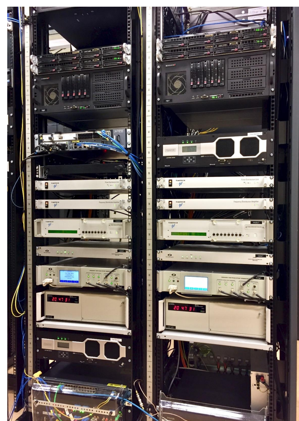
Figure 3. A time node, with cesium clocks (red displays), phase and frequency steppers (blue-white displays), distribution amplifiers, multi-channel time interval counters for monitoring, GNSS receiver, PTP grandmasters, and computers. The taller computers close to the top are the NTP servers.
