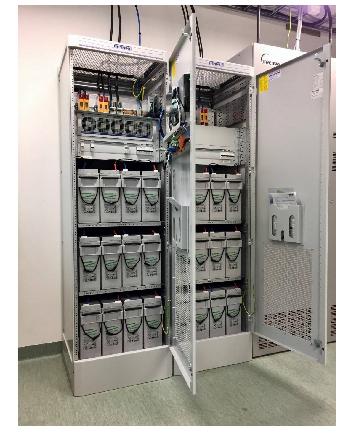
Figure 4. The time node sites have uninterruptible power supply such as battery UPS units and diesel generators. In addition, the time keeping equipment in the node has 24 VDC battery for another three days.
